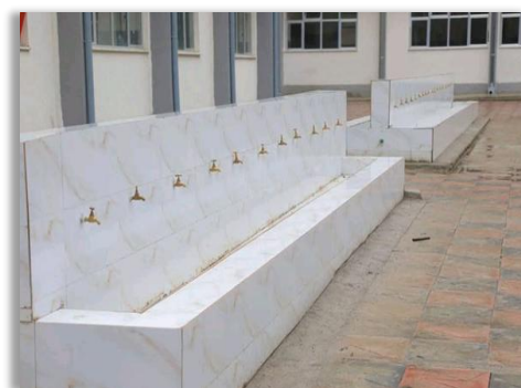
Water supply facility in school
